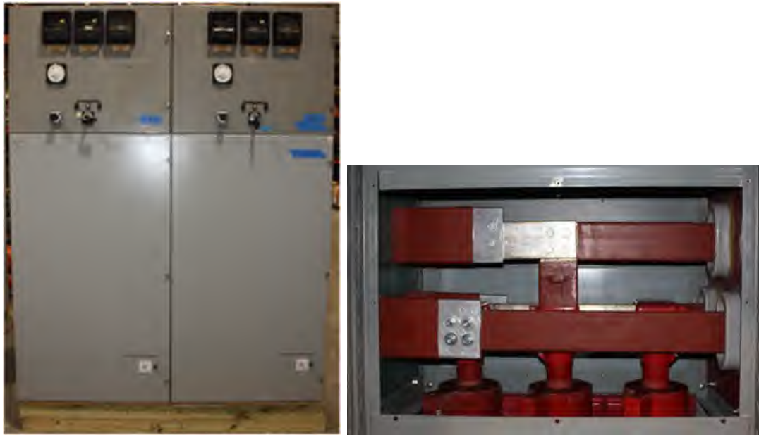
Fig. 189. Pre-Experiment 2-38 Enclosure “K” and “L”. Left - Enclosure “K” (left) and “L” (right), Right -arc location on main bus Enclosure “K”.
