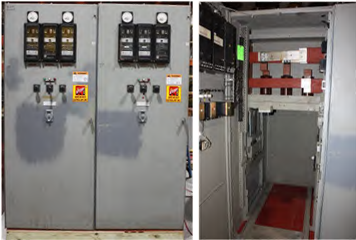
Fig. 178. Pre-Experiment 2-35 Enclosures “O” and “P”. Enclosure “O” (left) and “P” (right) front panel, Right – Inside Enclosure “O” showing main bus where arc was initiated.
