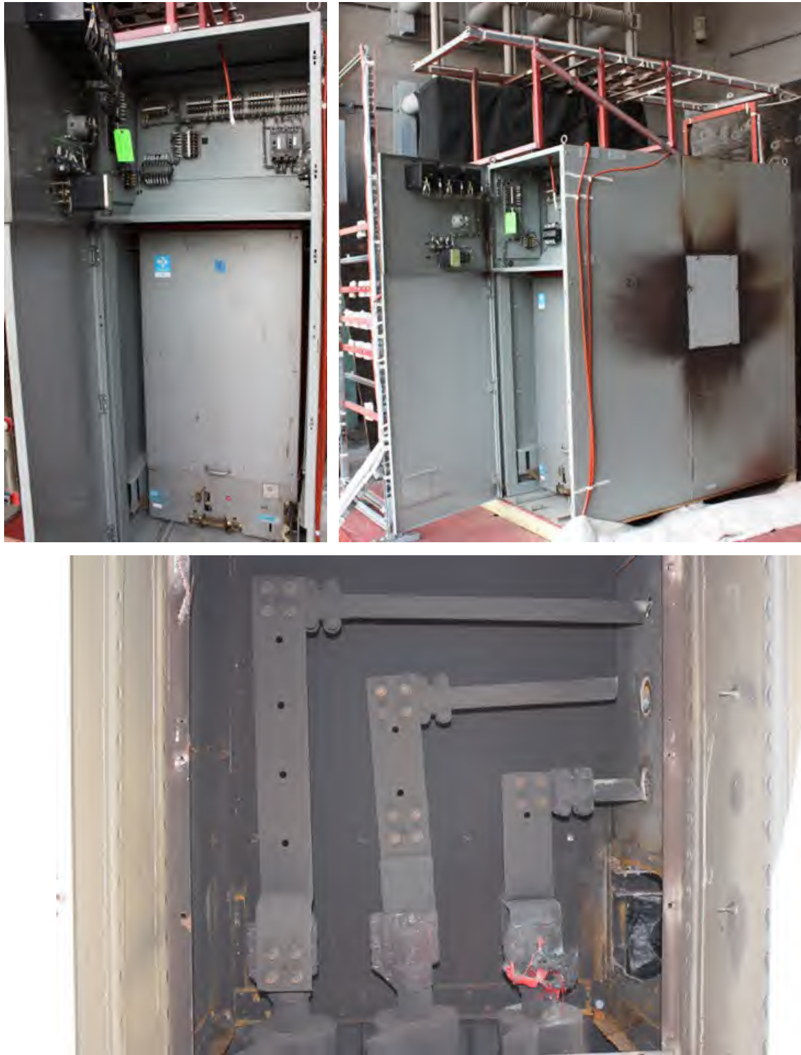
Fig. 184. Post-Experiment Enclosure "N". Top-left – front instrumentation and breaker cubicle, Top-right – side showing soot deposit near cover over main bus section of switchgear, Bottom – main bus section showing damage to horizontal copper bus.
