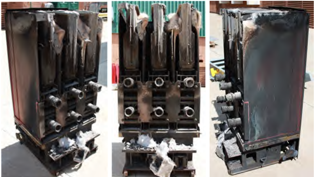
Fig. 199. Post-Experiment 2-37 Enclosure “M” Breaker. Left - rear angle view, Center – stab close-up, Right - rear angle view.
