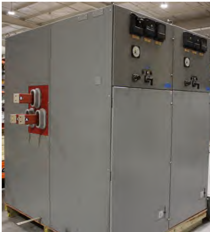
Fig. 9. Type M-36 Metal Clad Enclosure. Enclosure "J" shown left, "I" shown right. (note: bus bar extensions shown left, and breaker not shown)
