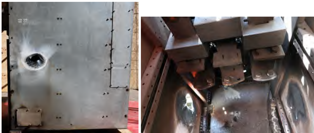
Fig. 215. Post-Experiment 2-XXA. Left – enclosure breach on right side of gear (cladding 1.5 mm [0.060 in] thick), Right – internal bus bar condition at arcing location.
