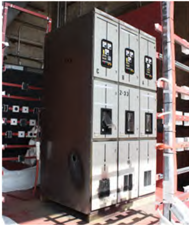
Fig. 162. Post-Experiment 2-33A. Note arc burn-through on side of Enclosure "C" (EV53), melting of vents in lower section and placement of breaker protection cover.
