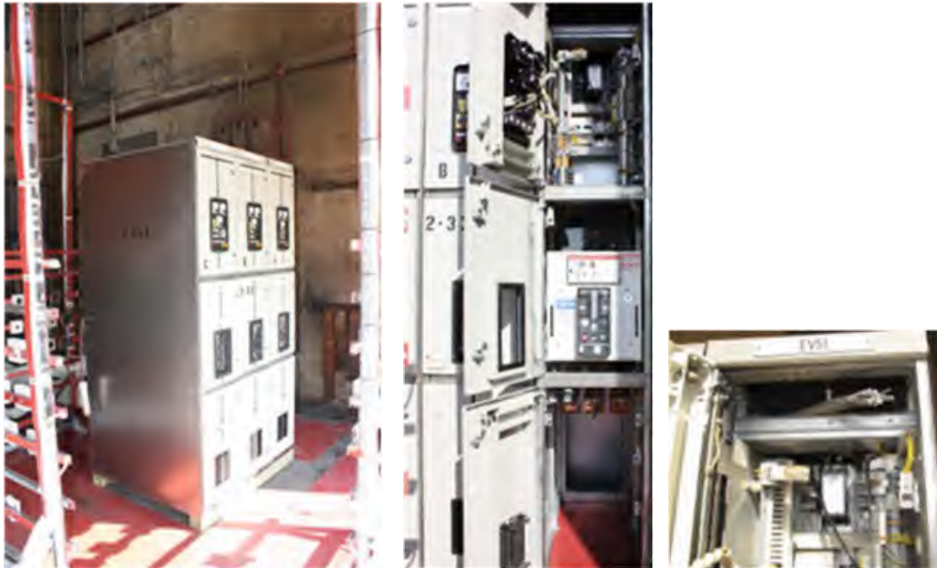
Fig. 160. Pre-Experiment 2-33A with equipment placed in Test Cell #7. Left – complete lineup, Center – Section 'A' internals viewed from front with doors open, Right – SIS wire pulled out to show amount installed in upper wire-way (note wire ends were pushed back into wireway prior to experiment).
