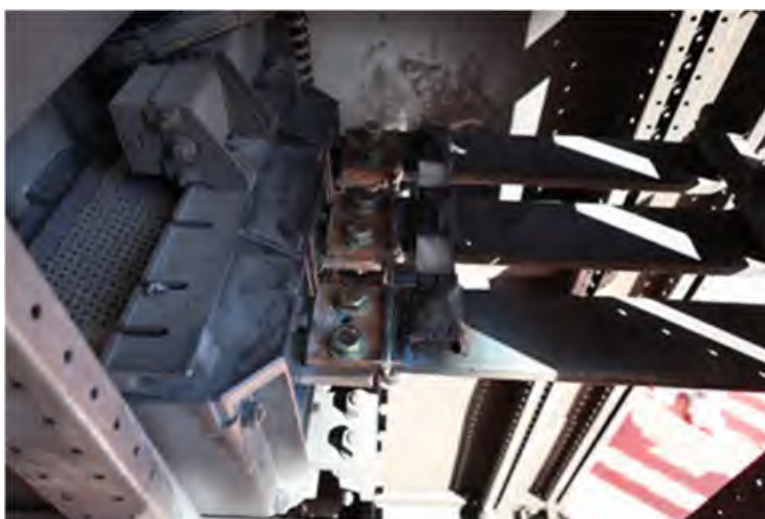
Fig. 216. Pre-Experiment 2-XXB. Arcing wire location.
