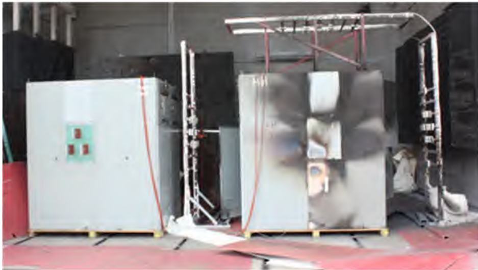
Fig. 192. Post-Experiment 2-38 Enclosure “M” and “L”. Front view of Enclosure “M” (left) with Enclosure “I” behind, and Enclosure “L” (right) with Enclosure “K” behind (where arc initiated).
