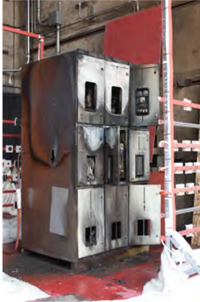
Fig. 37. Enclosures Post-Experiment 2-33B. Note the external breach on the middle side panel of Enclosure 'C'.
