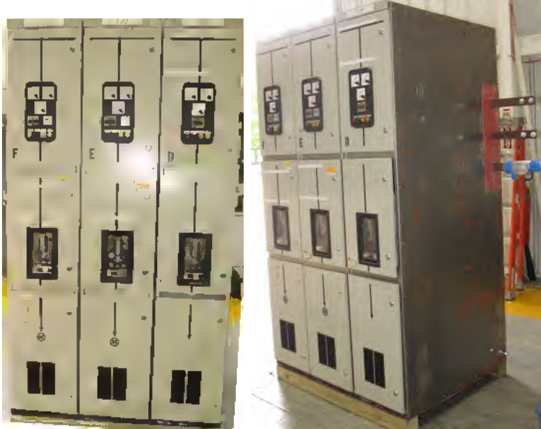
Fig. 17. Photographs of the low-voltage lineup configuration.
