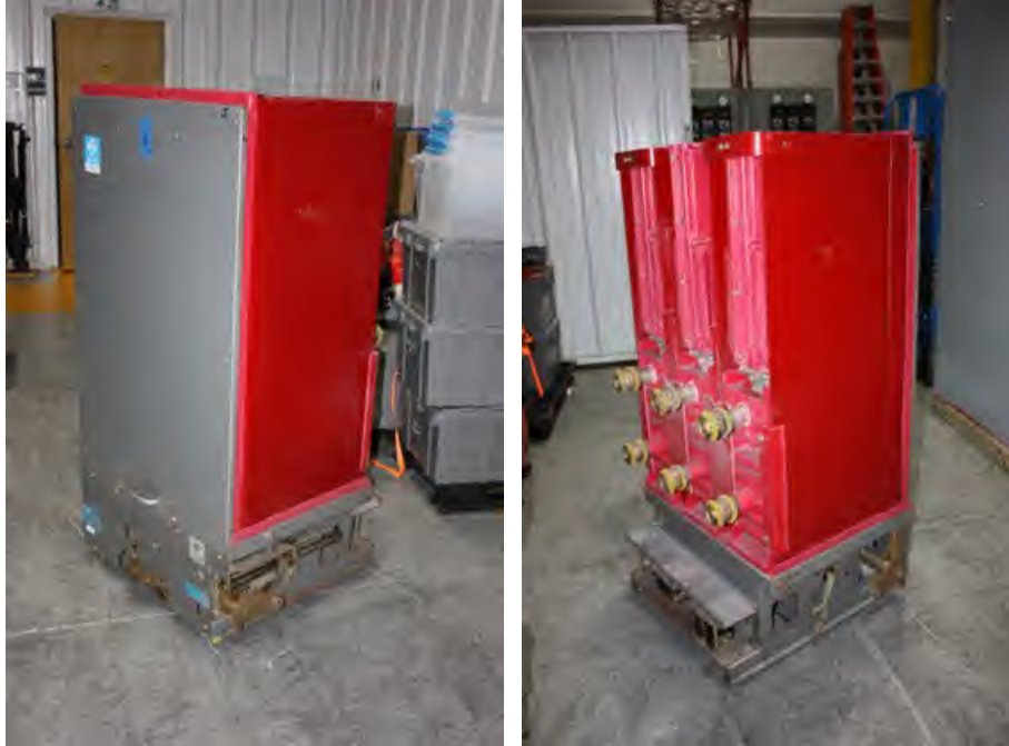
Fig. 11. Photo of GOULD I-T-E 7.5 HK-500 GE Magne-blast breaker
