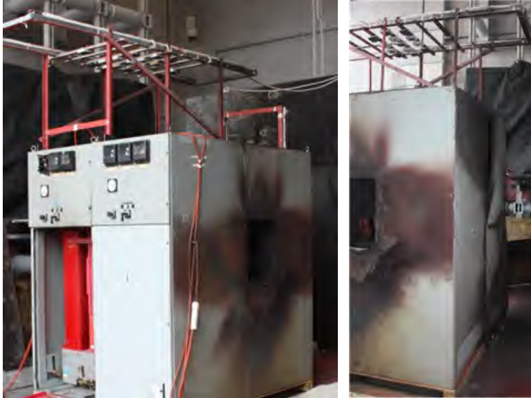
Fig. 63. Enclosure Post-Experiment 2-37. Door of Enclosure “J” was blown off, side panel of Enclosure “I” was blown off, and both rear panels were bowed.
