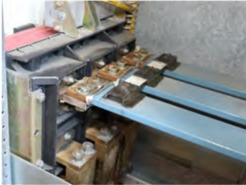
Fig. 219. Pre-Experiment 2-YYA arcing wire location.
