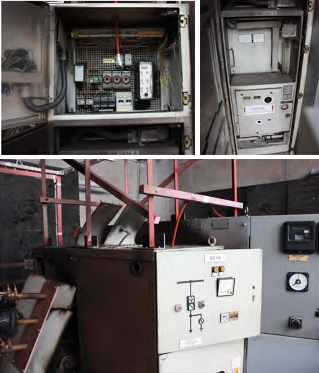
Fig. 183. Post-Experiment 2-36, Enclosure "H". Top-left – front instrument cubicle, Top-right – lower breaker cubicle, Bottom – exterior showing two panels re-oriented on top of enclosure, one panel on side completely disconnected from enclosure.
