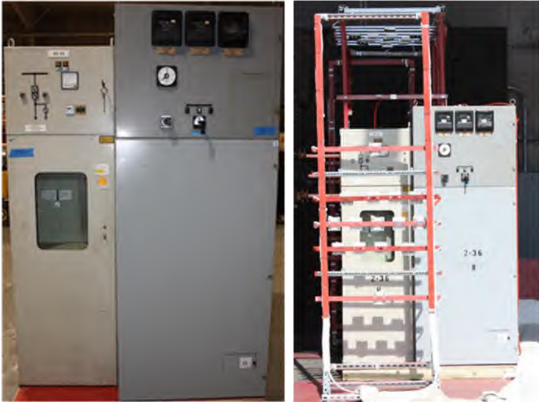
Fig. 182. Pre-Experiment 2-36 Enclosures “H” and “N”. Left – switchgear mockup at storage warehouse, Right – enclosures prior to experiment showing instrumentation rack locations.
