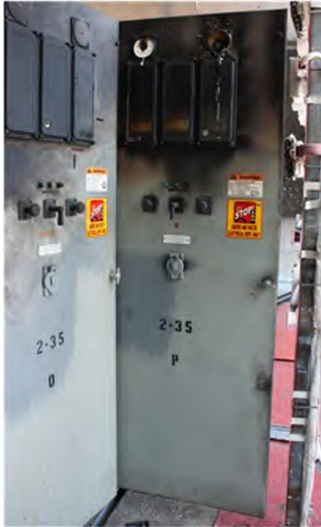
Fig. 180. Post-Experiment 2-35 Enclosures “O” and “P”. Soot and heat damage on front enclosure doors.
