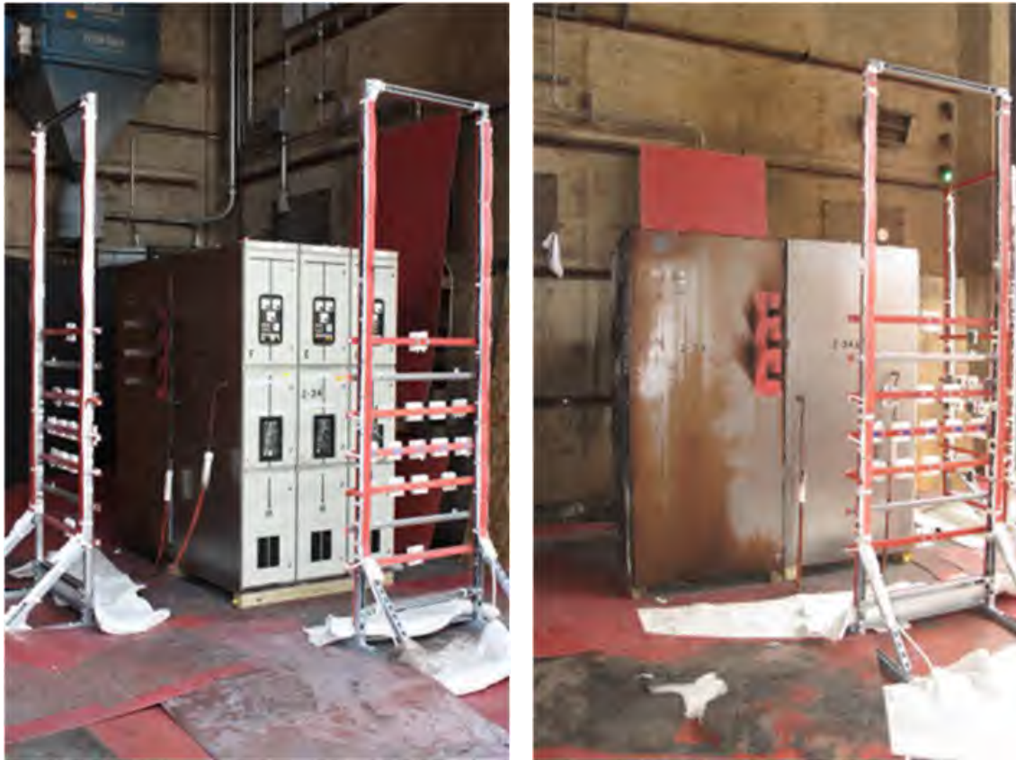
Fig. 174. Pre-Experiment 2-34 Enclosures “D”, “E”, and “F”. Left – front angle view of experimental device, Right – side view of “back-to-back” experimental configuration (note enclosure labeled 2-33 on left is not energized).
